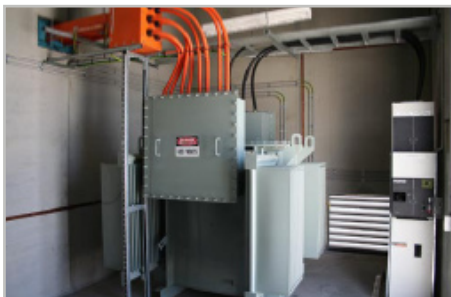
One of Two Step-Up 1000KVA Transformers supplying power to the refrigeration services.
