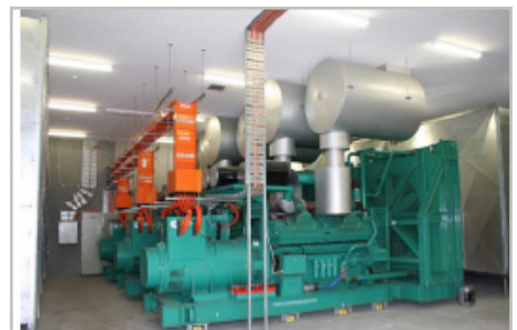
The Three 2,250KVA Generator sets supplying backup to the entire 42,000 square meter complex.
