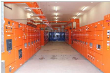
Main Switch Room supplying power to the 42,000 square meter warehouse.
